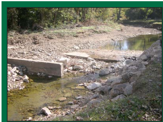
Concrete weir and concrete slab over 36-inch water main in Sweetbriar Park preconstruction
