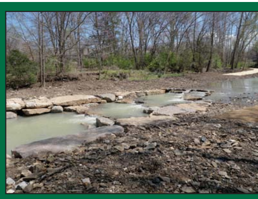
Vicinity of concrete weir and 36-inch water main in Sweetbriar Park after construction
